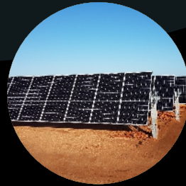
SOLAR ASSET LABELLING
